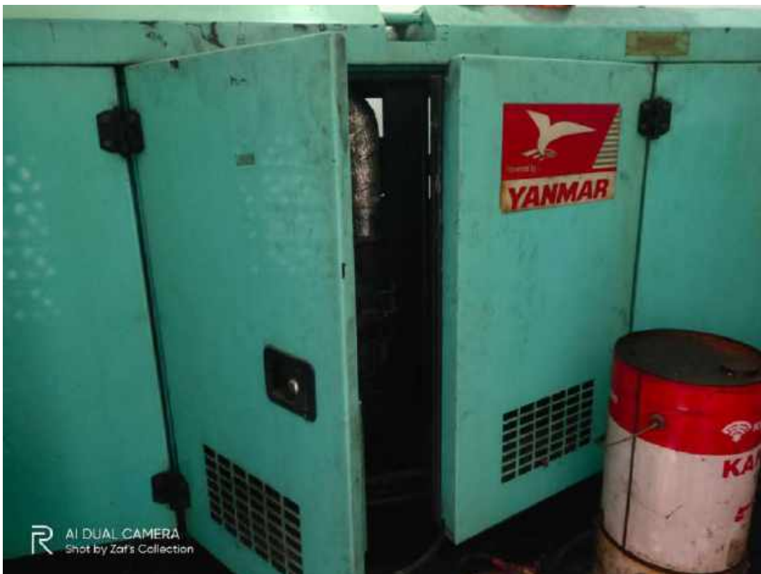
Lampiran 19. GENERATOR SET
